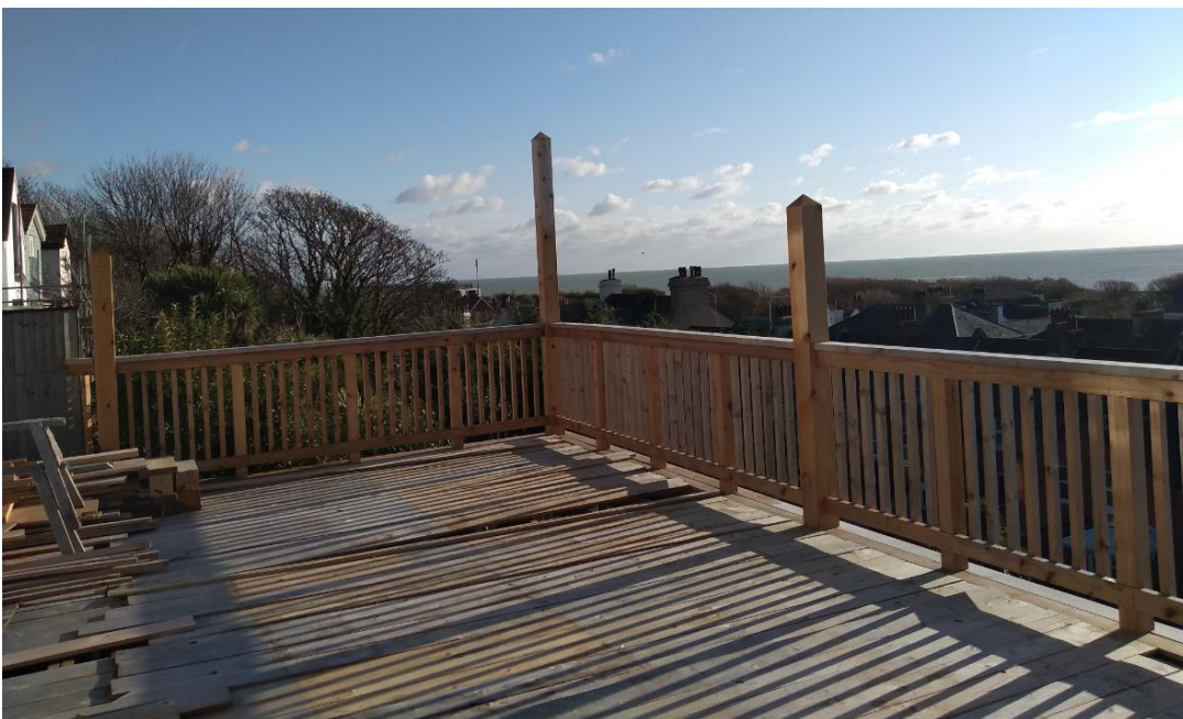
Figure 6: evidence of unfinished works
